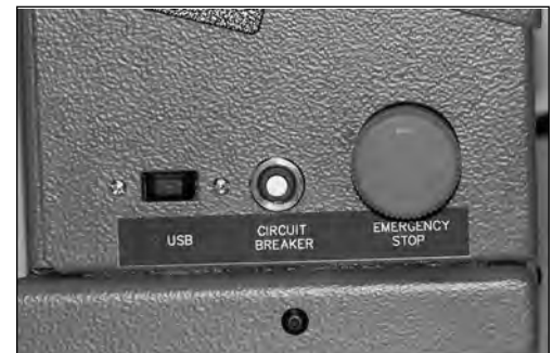
Side view of Main Circuit Box
